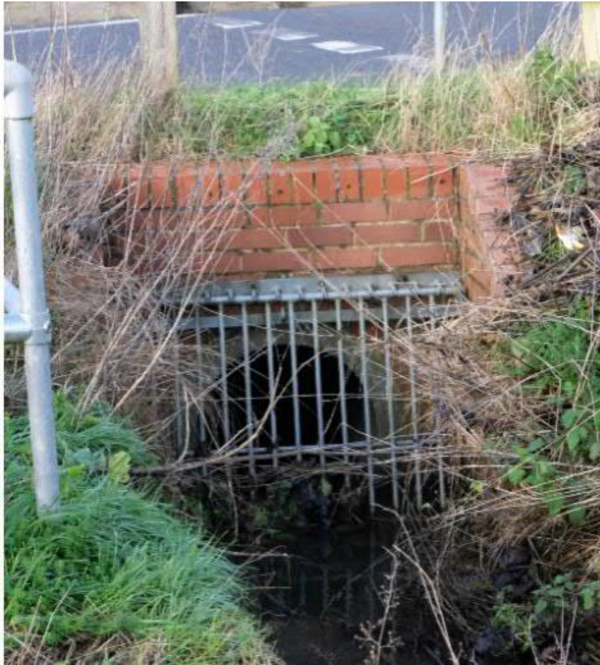
Figure 11: Culvert in Shudrick Lane, taken some time after the incident.
