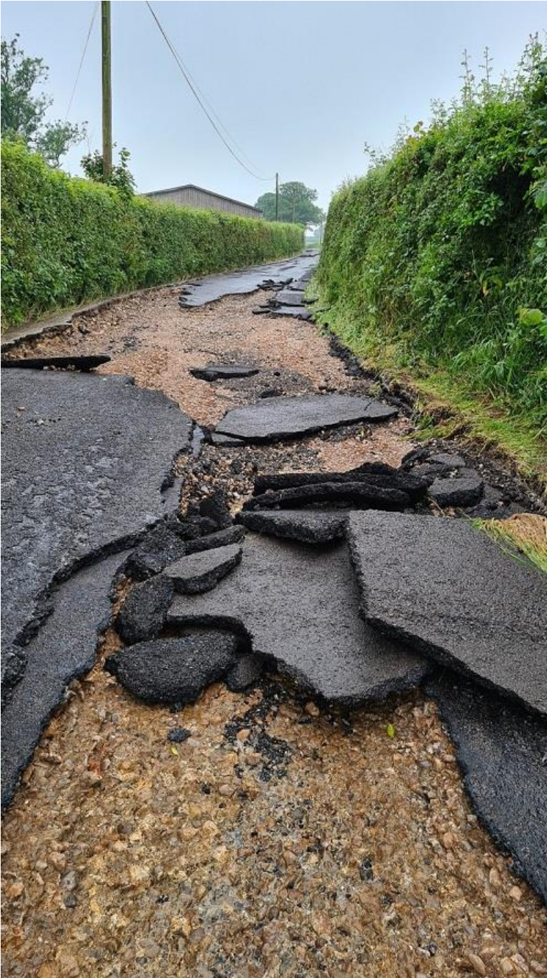
Figure 35: Road damage in Whitestaunton. Photo from Access restored as Highways teams respond to flash flooding damage | Somerset County Council Newsroom ( somersetnewsroom.com ).
